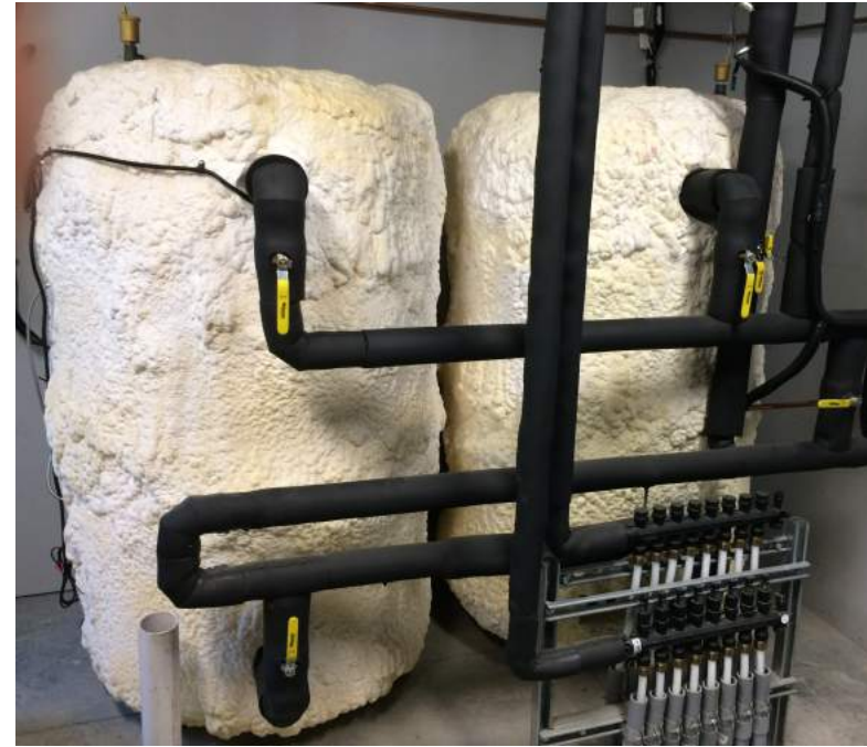
2 coupled pressurized tanks
